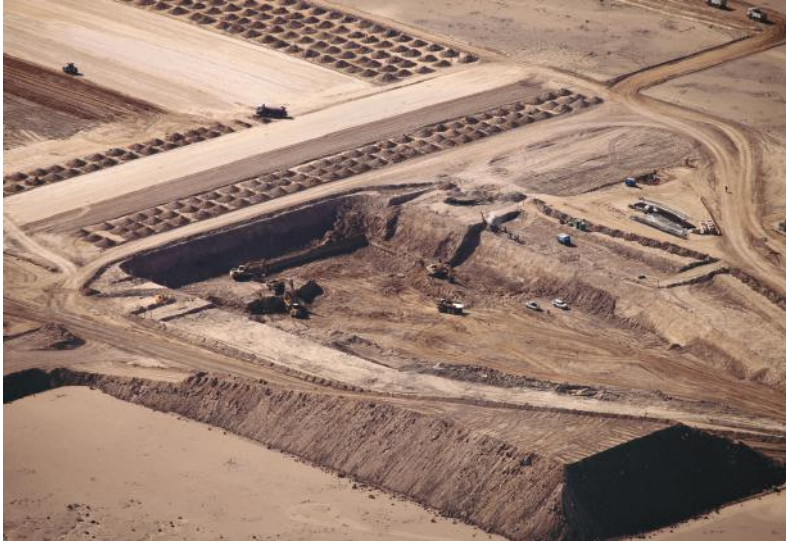
PROGRESS: An aerial picture of construction activities on the Husab project site
