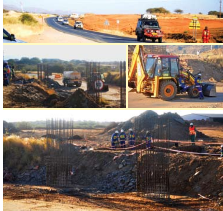
MEGA ROADWORKS: Construction work on the B1 Highway between Windhoek and Okahandja is in full swing, with the four-lane dual carriageway between the two centres being extended from Brakwater right up to Okahandja
