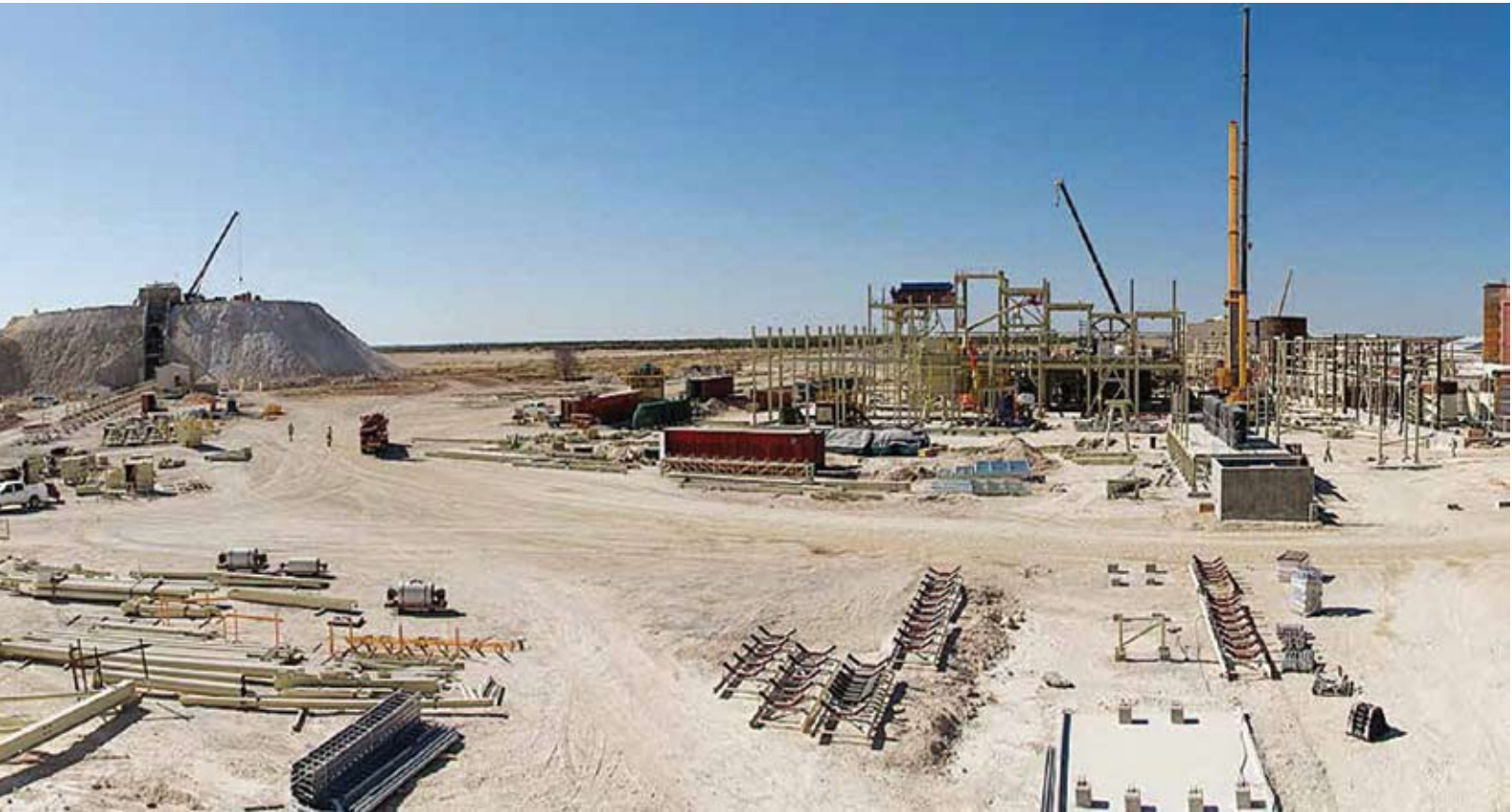
ON TRACK: Construction of the Otjikoto mine remains on schedule to commence gold production in late 2014 Photo: Courtesy of Chamber of Mines
