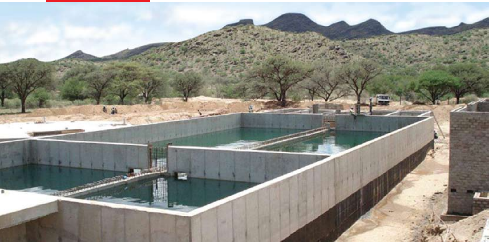
The Gammas Water Reclamation Plant
